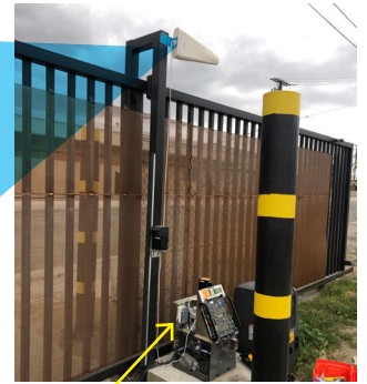
Cell Hub behind a gate with metal mesh
