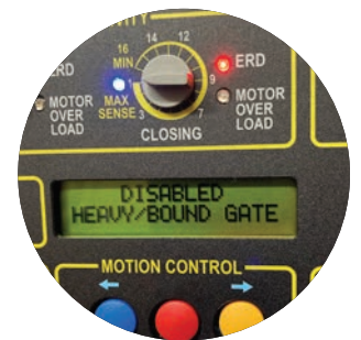
Heavy gate or binding gate detected
